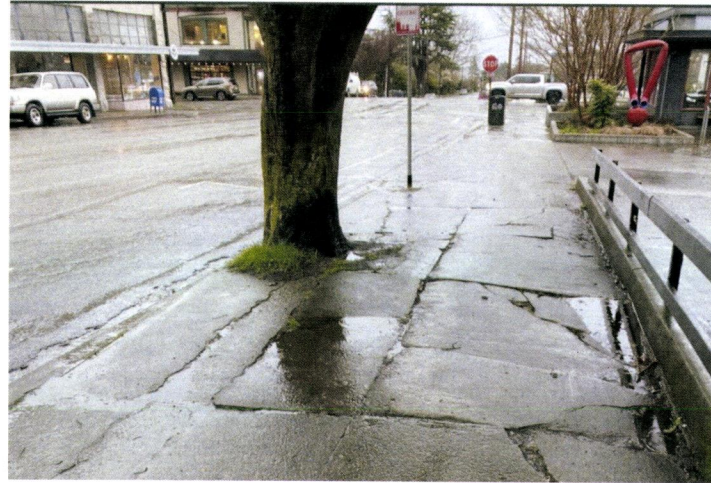
Sidewalk heaving around street tree
