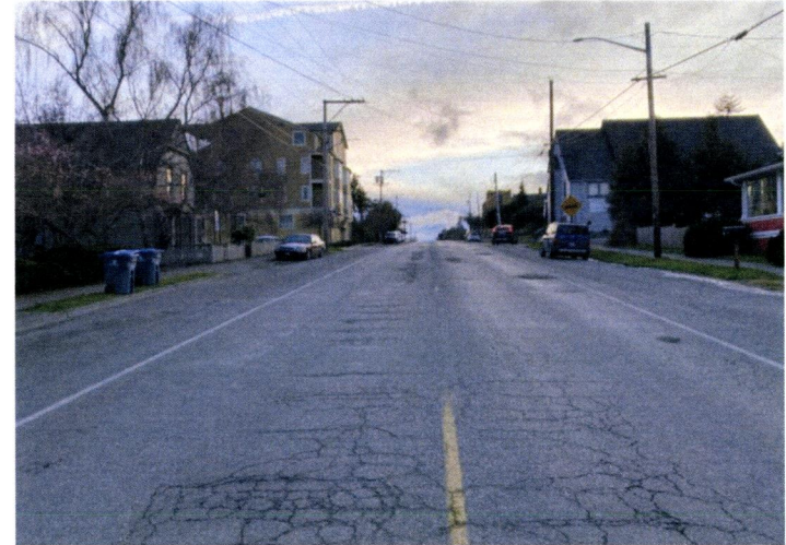
Existing pavement failures to be repaired with a storm/sewer separation project and future pavement project
