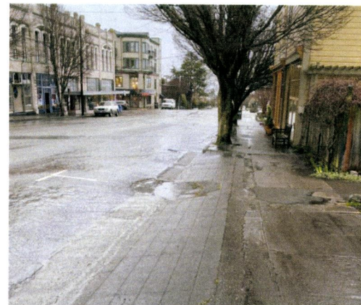
Existing driveway that needs to be removed along with damaged sidewalk
