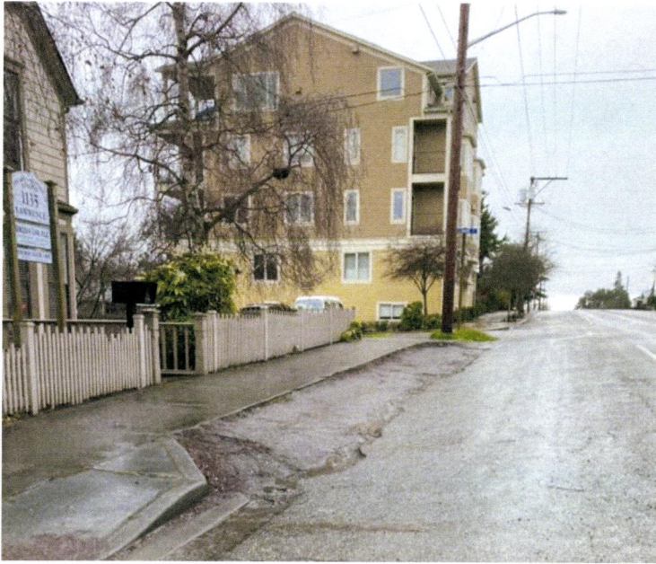
Missing sections of curb
