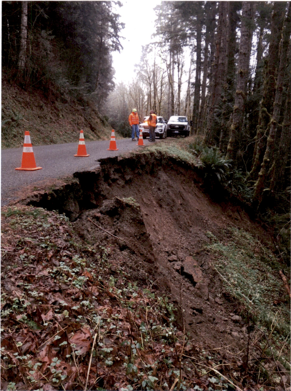
Lords Lake Road – Still Awaiting FEMA Construction Funding 6 Years Later
